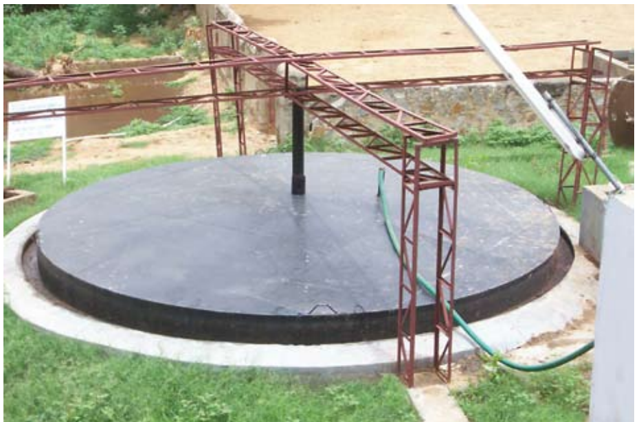
A biogas plant at IIT Delhi's Centre for Rural Development & Technology
